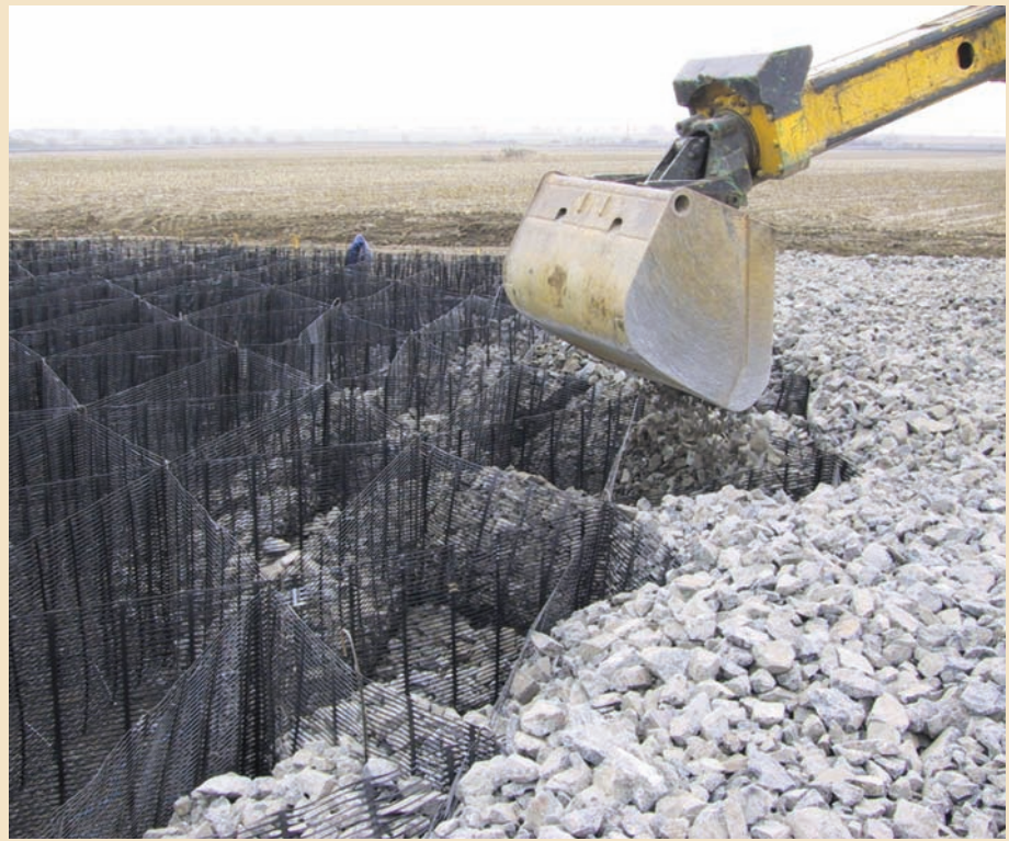
3. Approved fill is carefully machine placed into the cells and requires no compaction
