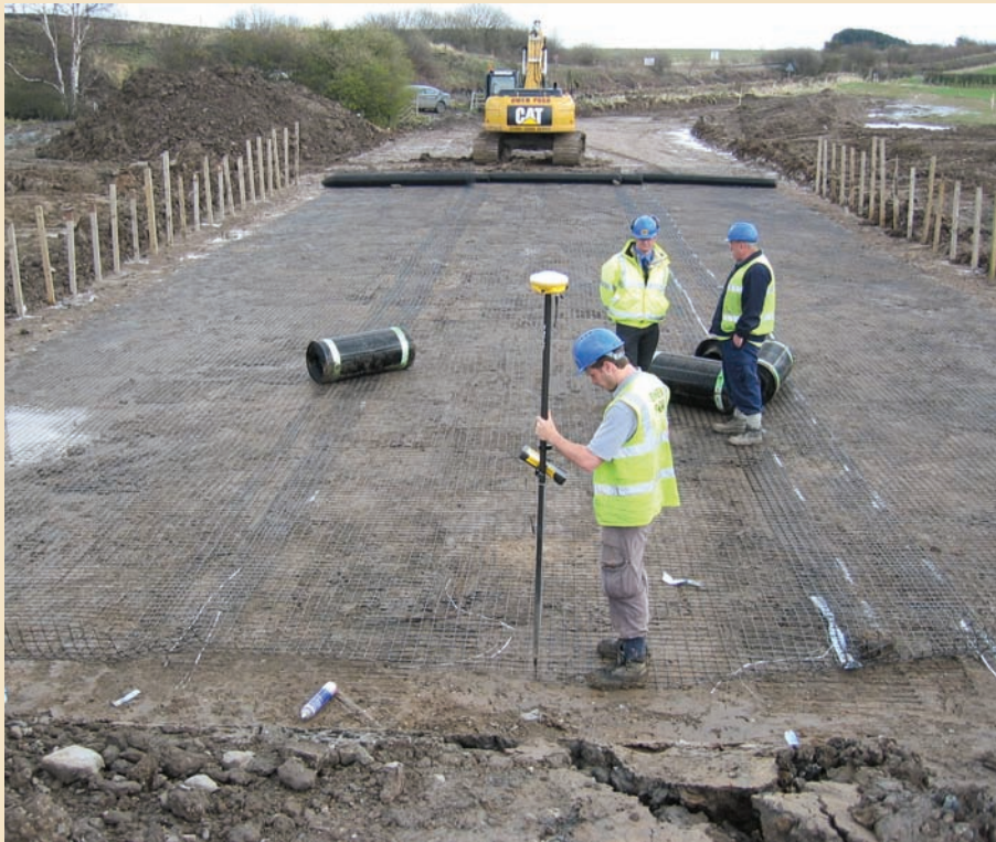
1. The base of the Geocell is quickly formed by unrolling geogrids onto the formation
